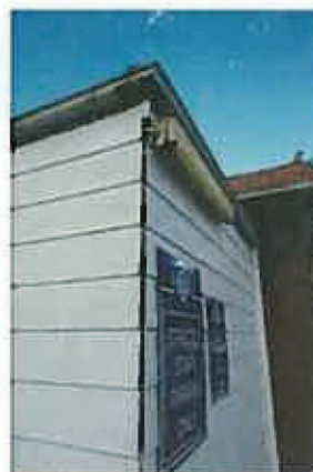
Figure 45: Front south-west corner of enclosed verandah, showing deteriorated guttering
